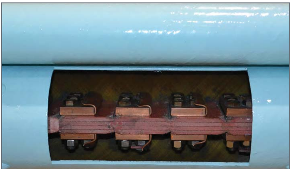
▲ Close up of the severed main conductor and melted current limiting element of a 3000A (double bus) CLiP after interruption.
